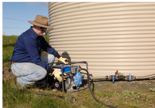
Test the pump regularly prior to and during the fire danger season.
